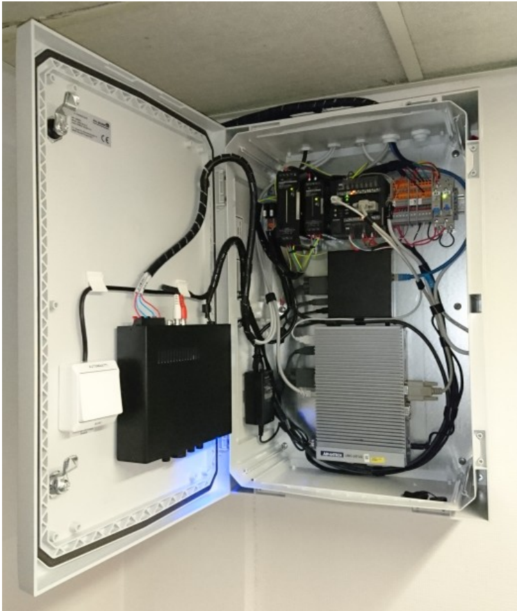
Main controller - inside
